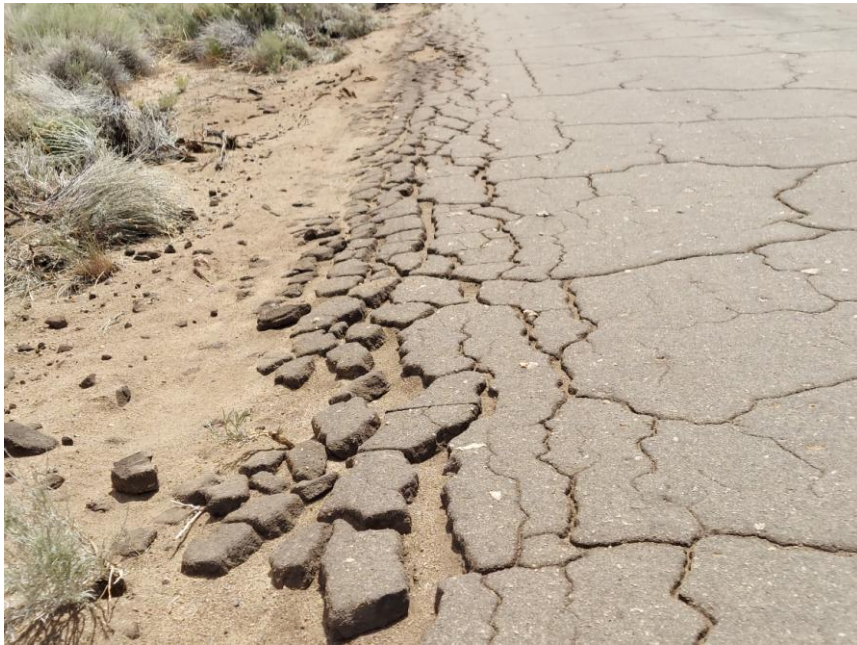
Right Hand Canyon Road Old, deteriorating pavement.
