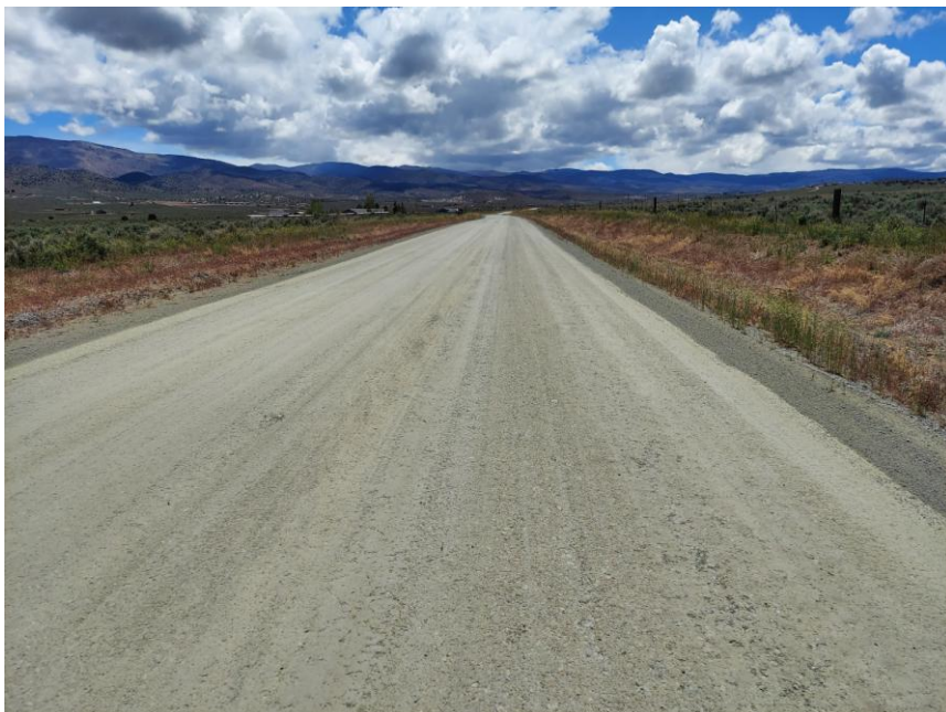
Range Land Road Covered deteriorating Cape seal with Class E base and applied mag- chloride.
